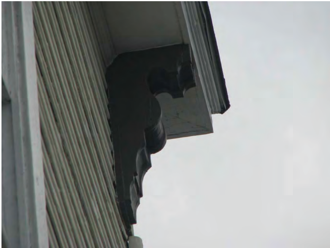
Restovich House, roof corbel, 1001 Everett Street, September 19, 2014 (Photograph by Charles J Fisher)
