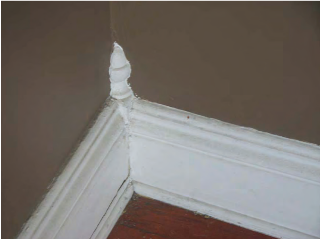
Restovich House, baseboard, 1001 Everett Street, September 19, 2014 (Photograph by Charles J Fisher)
