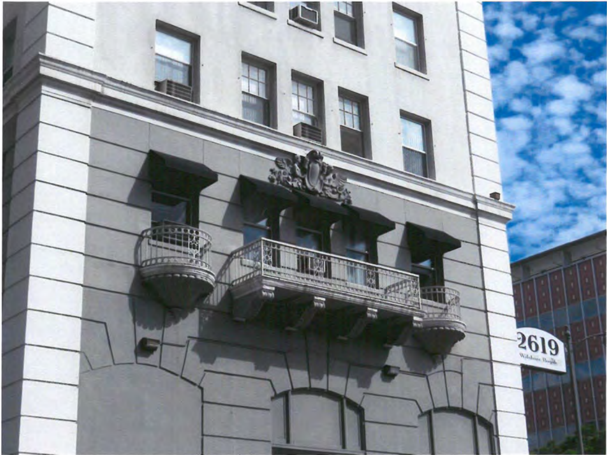
Detail, second story balcony, west façade, (southern wing). Note balcony and railing details, and oriel balconies with decorative base, and cast stone ornament.
