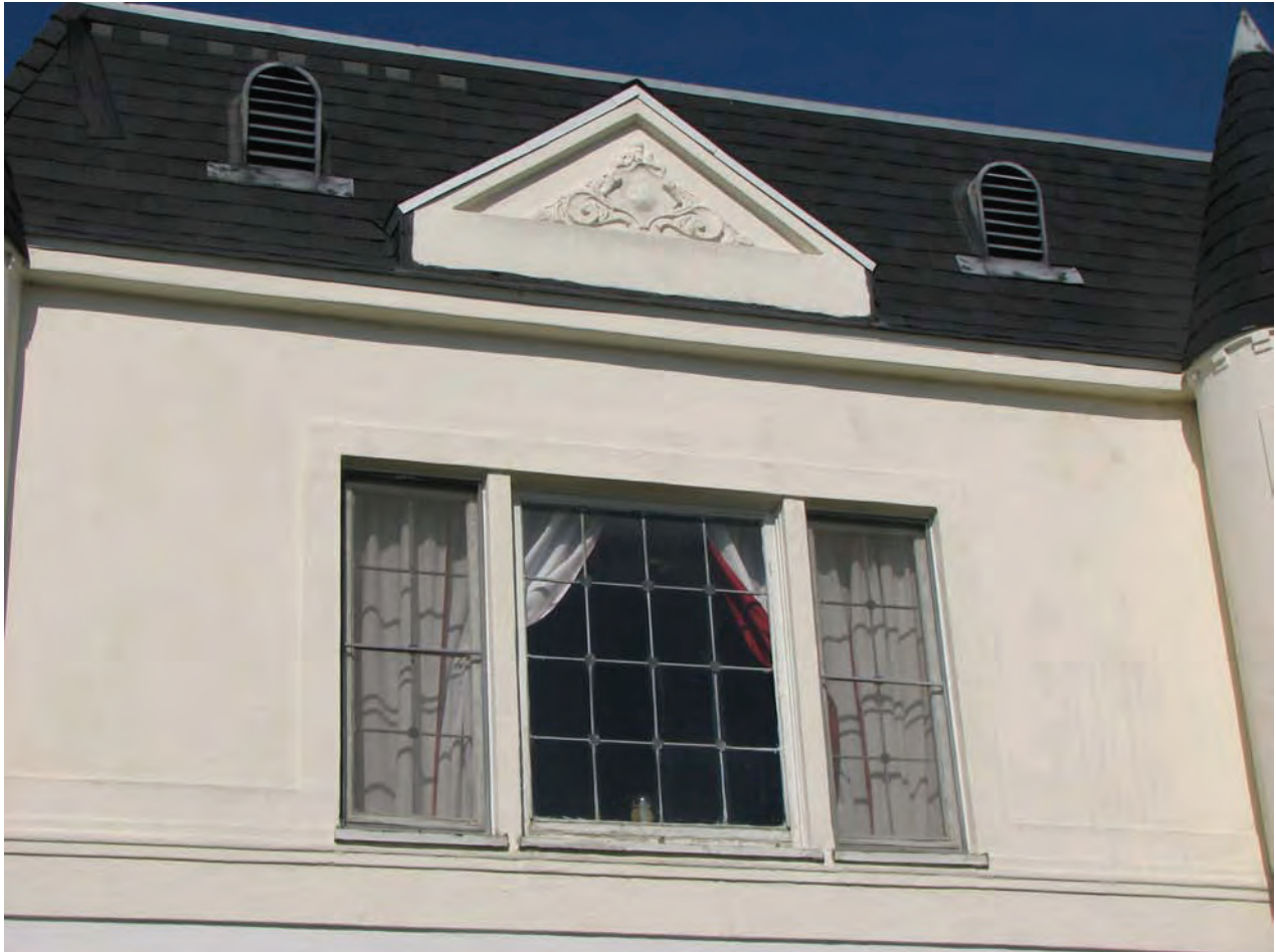
Spinning Wheel Apartments, 423-27½ N. Hayworth Avenue, April 12, 2016 (photograph by Charles J. Fisher)
