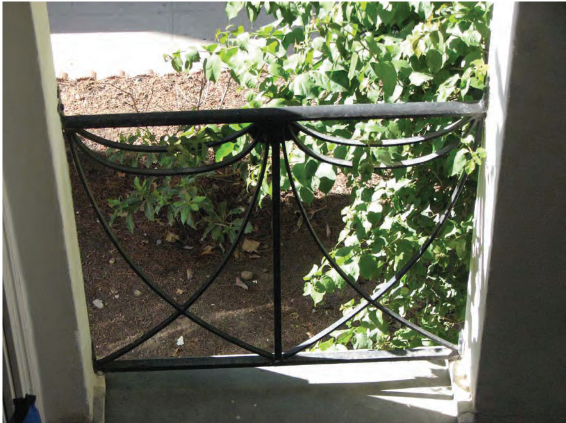
Spinning Wheel Apartments, railing, 423-27½ N. Hayworth Avenue, April 12, 2016 (photograph by Charles J. Fisher)
