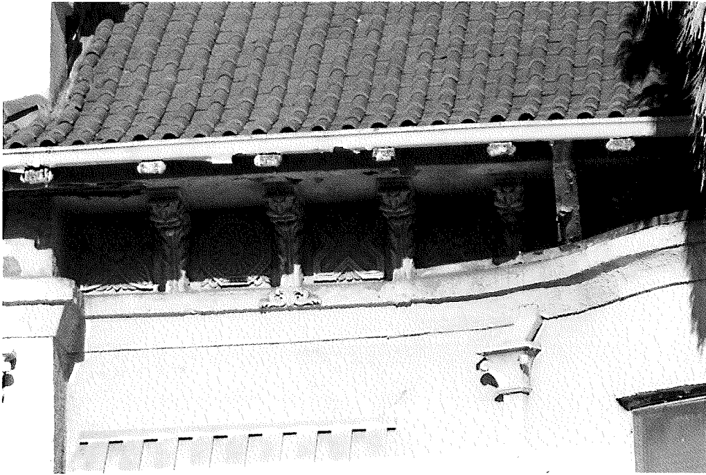
Details: Gutter brackets, eaves with decorative brackets with decorative plaques between them. Decorative member on banding. Decorative members on downspout headers.
