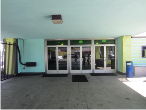
Primary opening on West Elevation Underneath Porte-Cochère, (Doors are replacements, date unknown and security gates to north are additions, date unknown), View East
