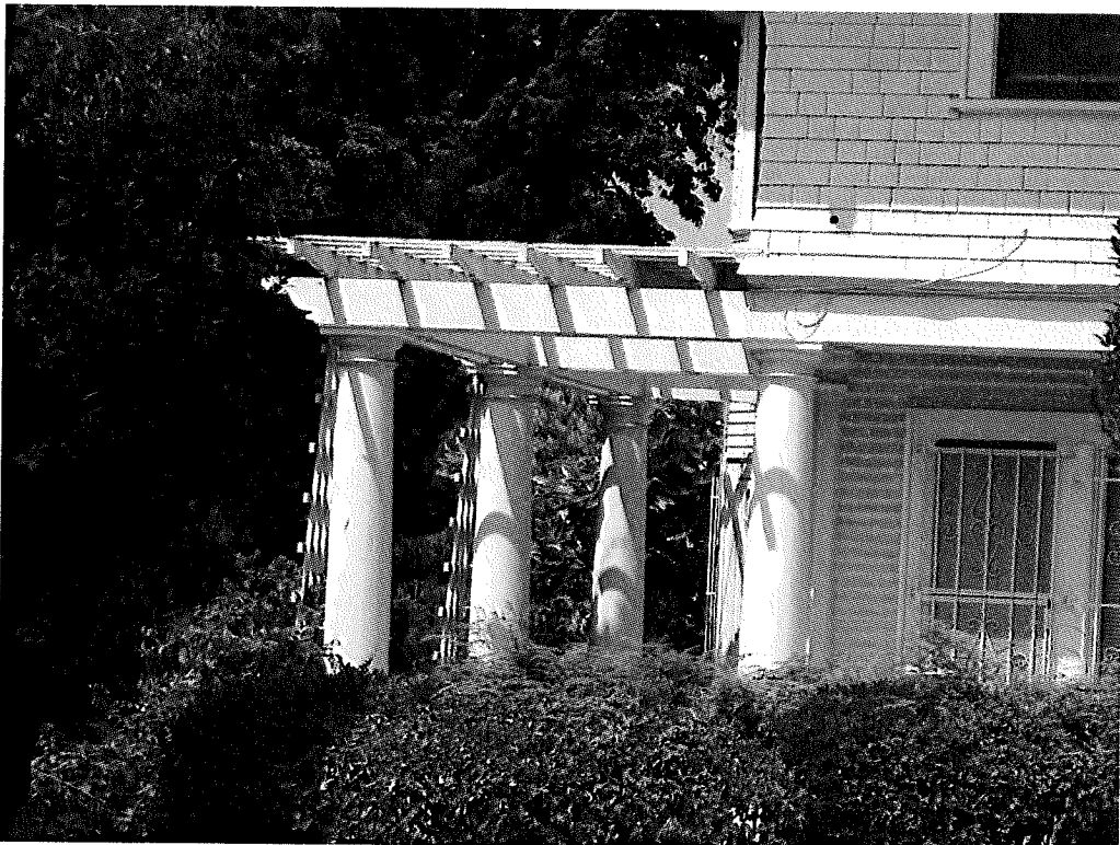
Bartlett Residence, pergola on South facade, 1829 N. Kenmore Avenue, August 7, 2014 (Photograph by Charles J. Fisher)
