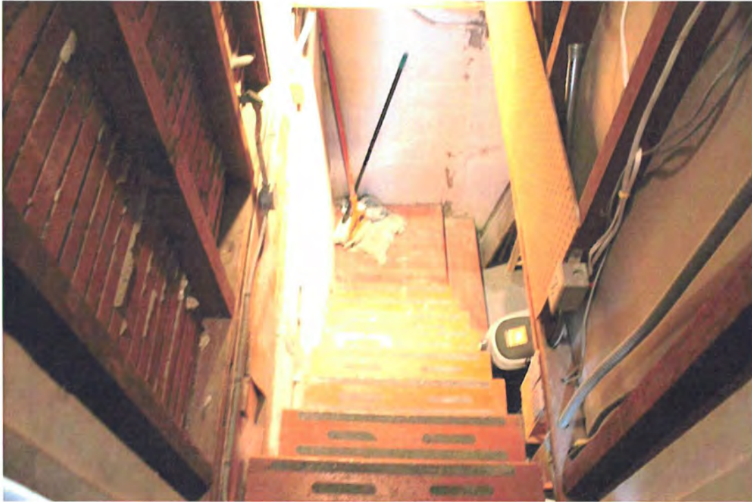
Cellar: West wall; stairs down to landing at north wall, view north.
