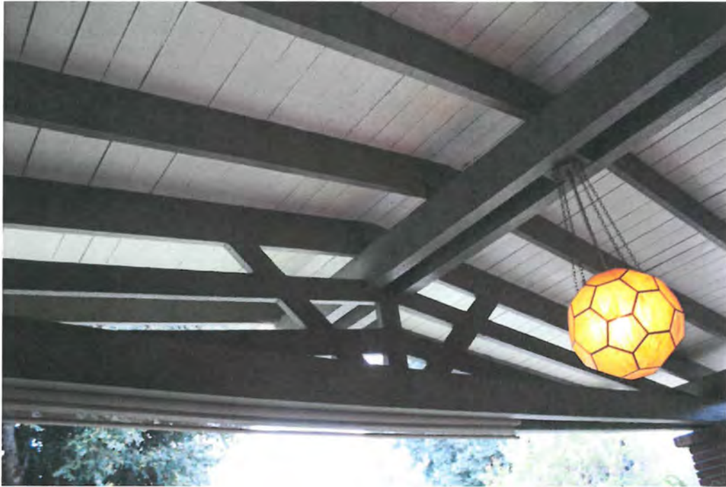
West porch interior gable configuration: Beamed, tongue & groove porch ceiling, view northwest.
