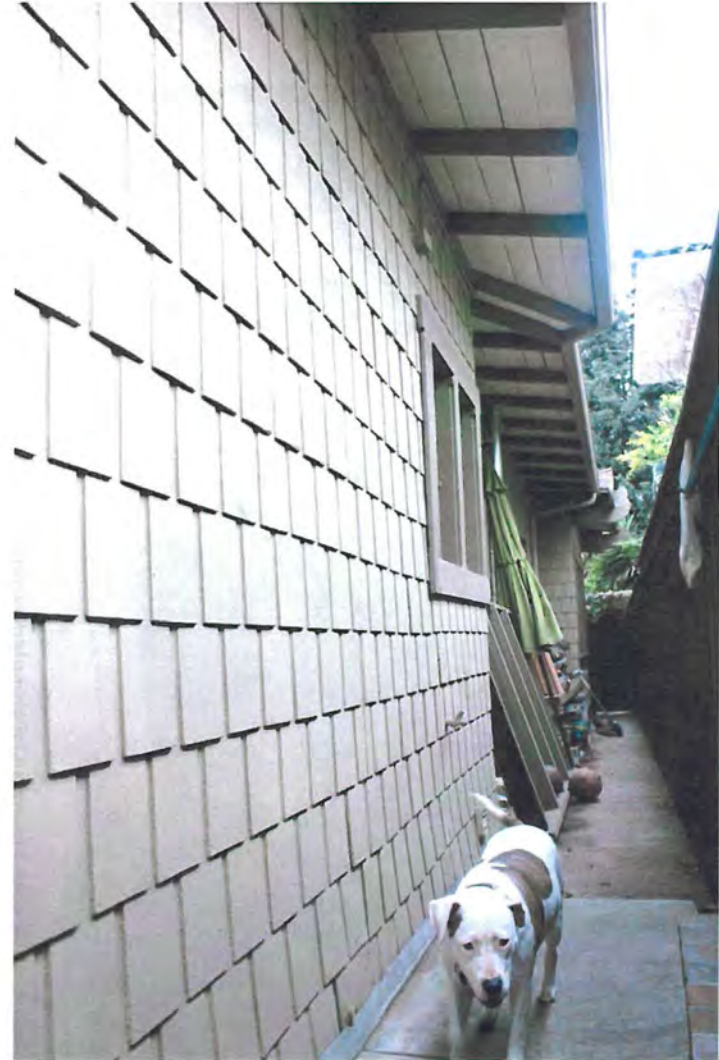
North shingled elevation, viewed west: Eaves with enclosed beam ends, at west Oriental gable with Oriental beam ends.
