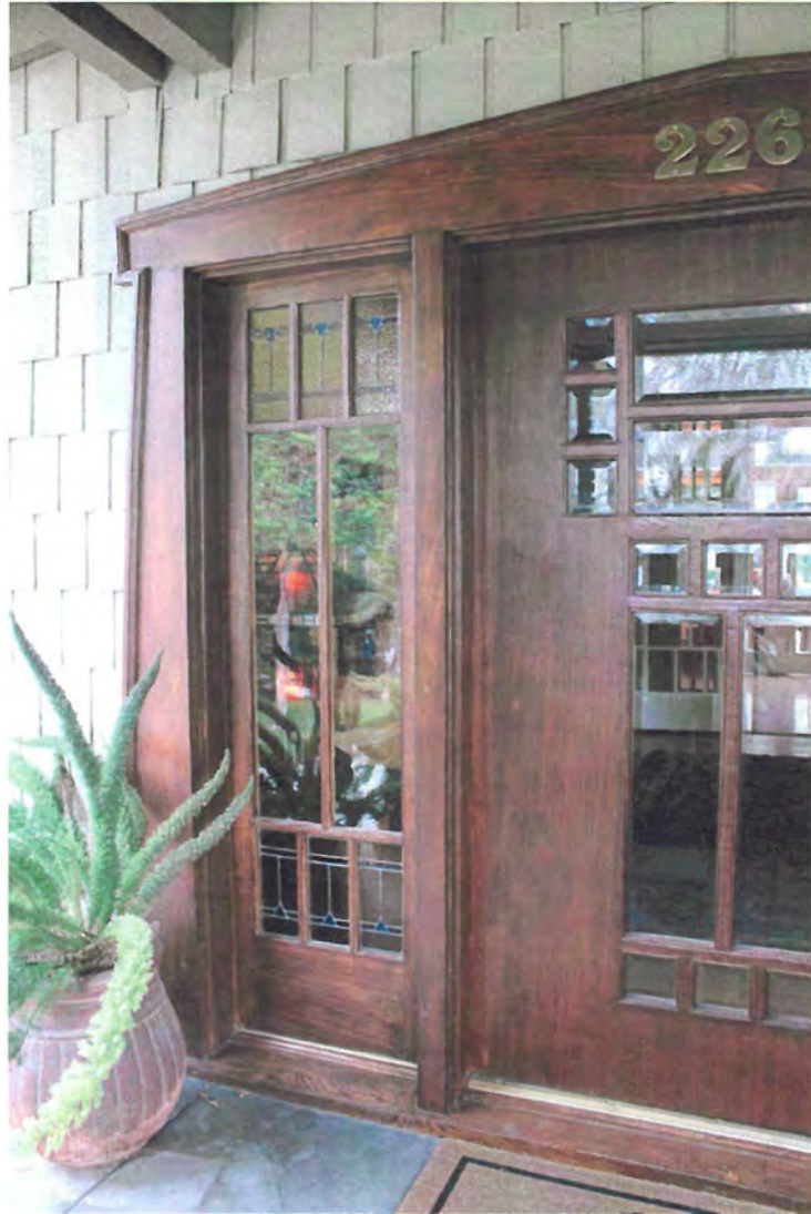
Entry: Sidelight with leaded art glass panes and plain glazing; partial entry door from west raised porch, view east.
