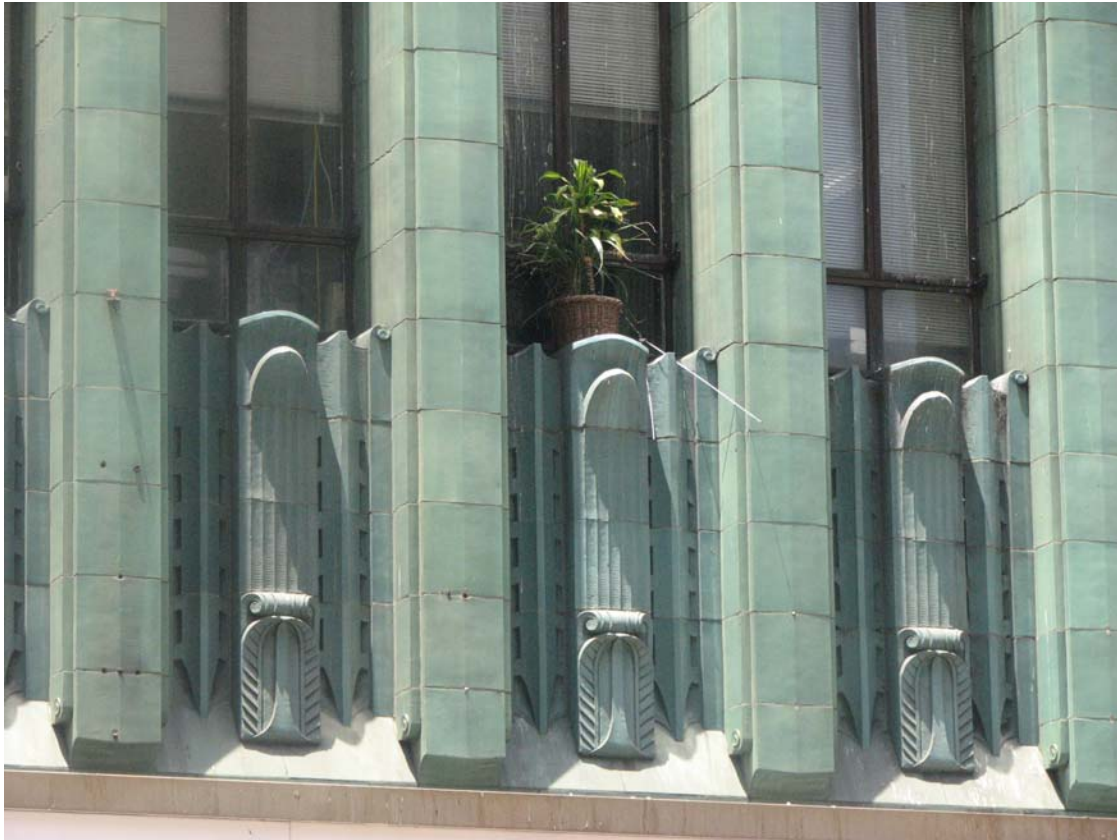
Sun Realty Company Building 2 nd floor terra cotta, 629-33 S. Hill Street, June 2, 2009 (Photograph by Charles J. Fisher)
