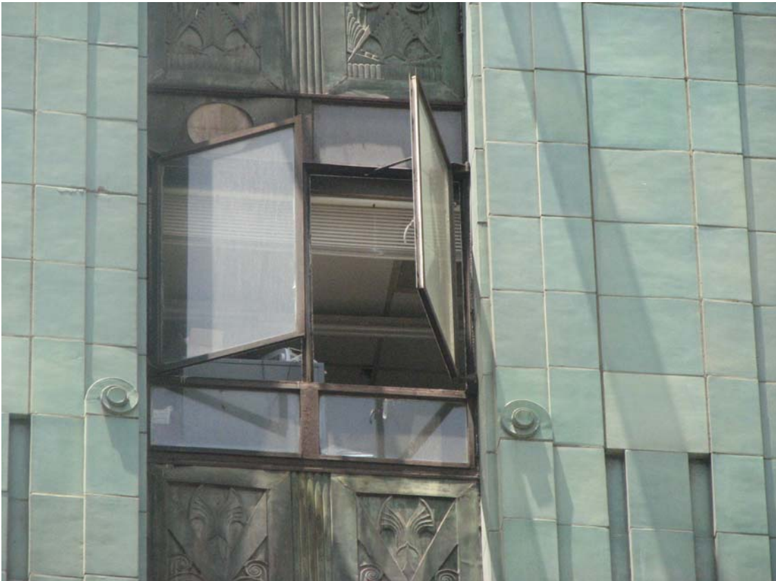
Sun Realty Company Building, casement window in front facade, 629-33 S. Hill Street, June 2, 2009 (Photograph by Charles J. Fisher)
