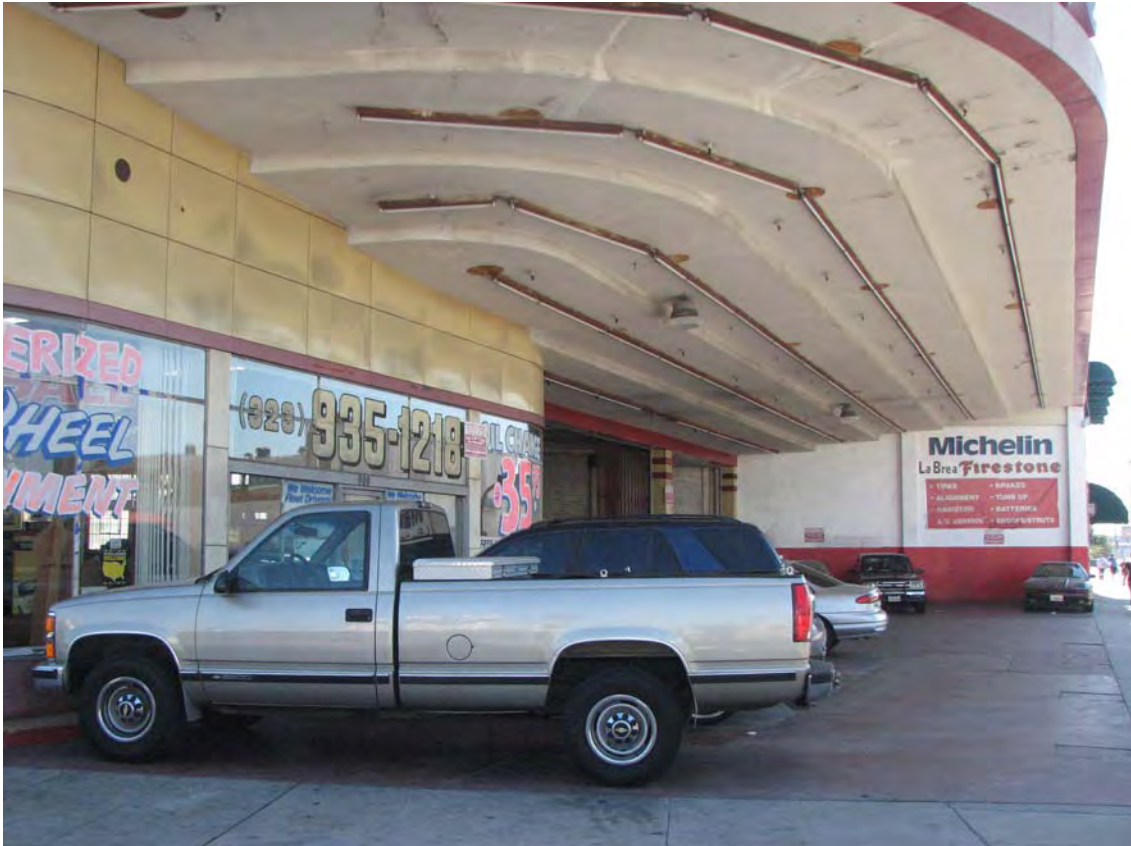
Firestone Tire Building, roof canopy, 800 S. La Brea Avenue, October 29, 2011 (Photograph by Charles J. Fisher)
