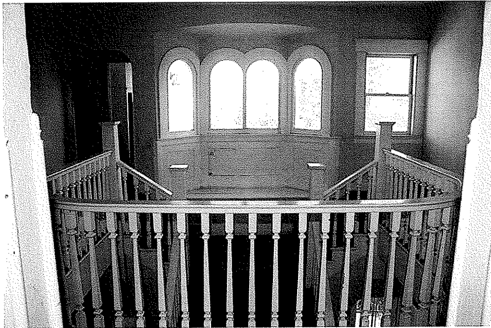
View of second level hallway, to east. Photo: February 2009 ~ © Anna Marie Brooks 2009
