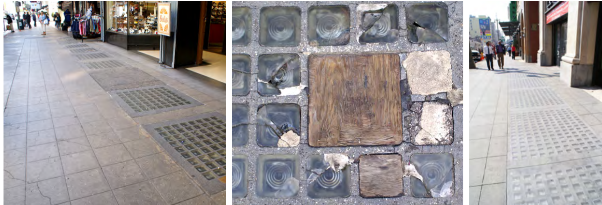
Glass Block Basement Skylights provide daytime illumination to basements below. Many are in need of critical repair and restoration.
