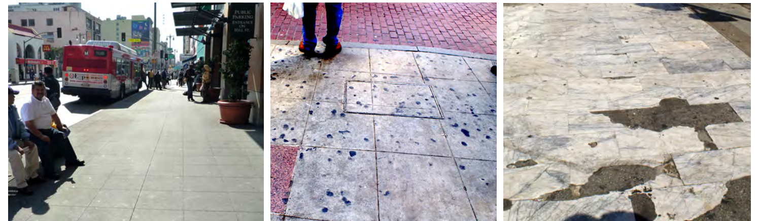
Some Sidewalk paving along Broadway has been laid in recent years, other shows its age. Other materials aside from concrete have been used, and are patched with asphalt.
