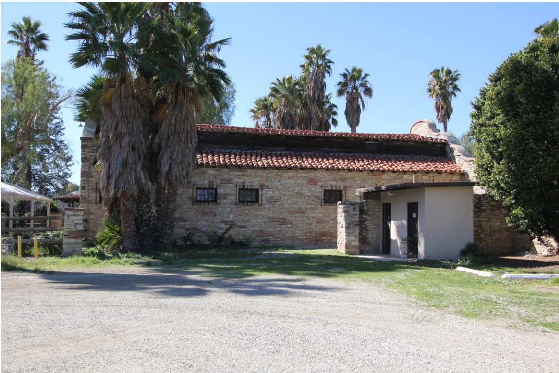
Figure 13: View showing the break in the roof line that roughly corresponds to the second floor attic space, view west, 2016 (Chattel, Inc.)
