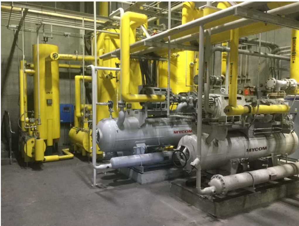
Chiller equipment room at east end of subject property. 1570 Industrial Street, Los Angeles, CA 90021
