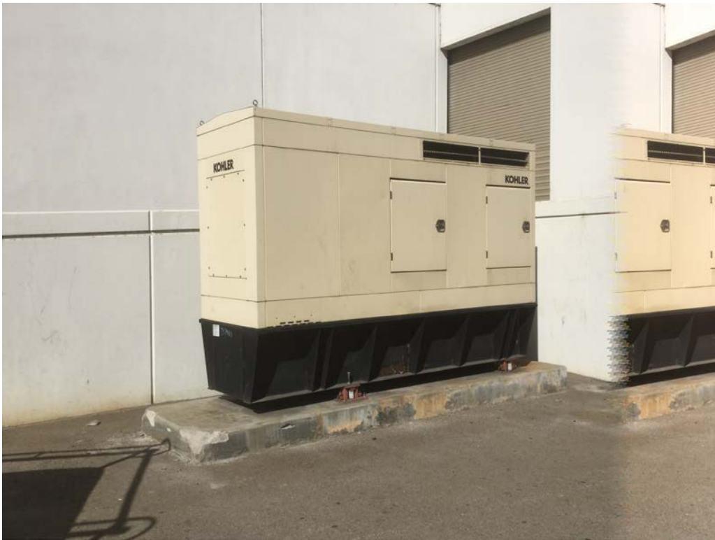
Aboveground storage tank and backup generator for subject building 1570 Industrial Street, Los Angeles, CA 90021
