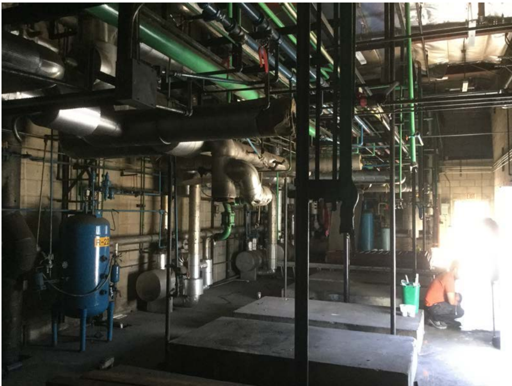
Former chiller equipment room at west end of subject property. 668 Alameda Street, Los Angeles, CA 90021
