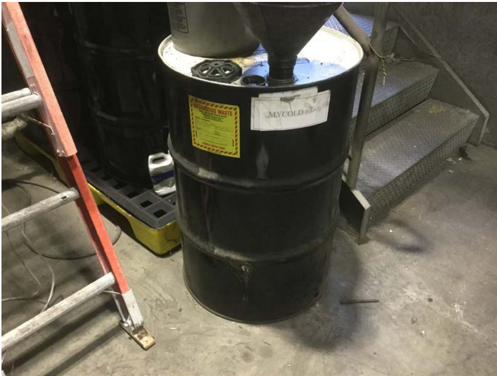
55-gallon drum of refrigerant in chiller equipment room at east end of subject property. 1570 Industrial Street, Los Angeles, CA 90021
