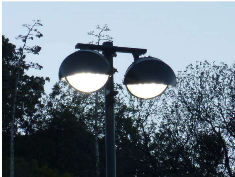
Existing Musco Fixtures
