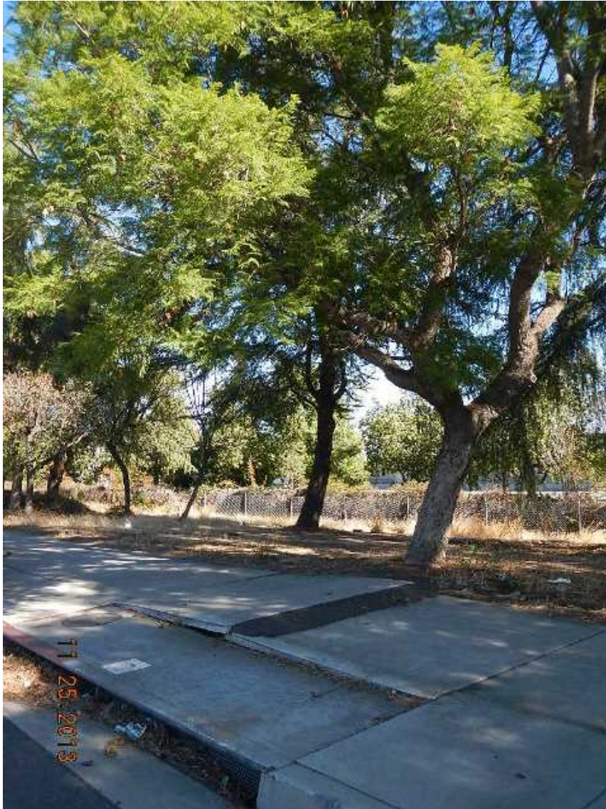
This larger jacaranda is lifting the sidewalk.
