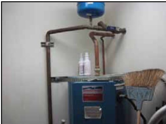
41 : Typical electric water heater
