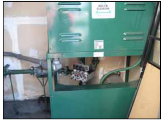
32 : Typical elevator equipment
