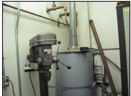
42 : Typical natural gas water heater
