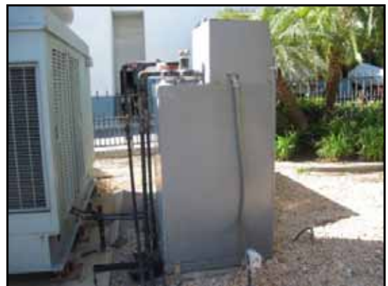
36 : Generator day tank
