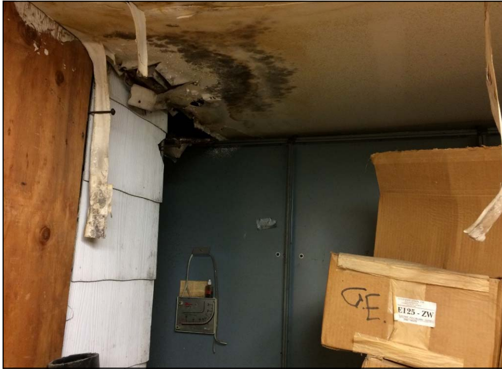
Photo 23: View of suspect mold growth within storage building.
