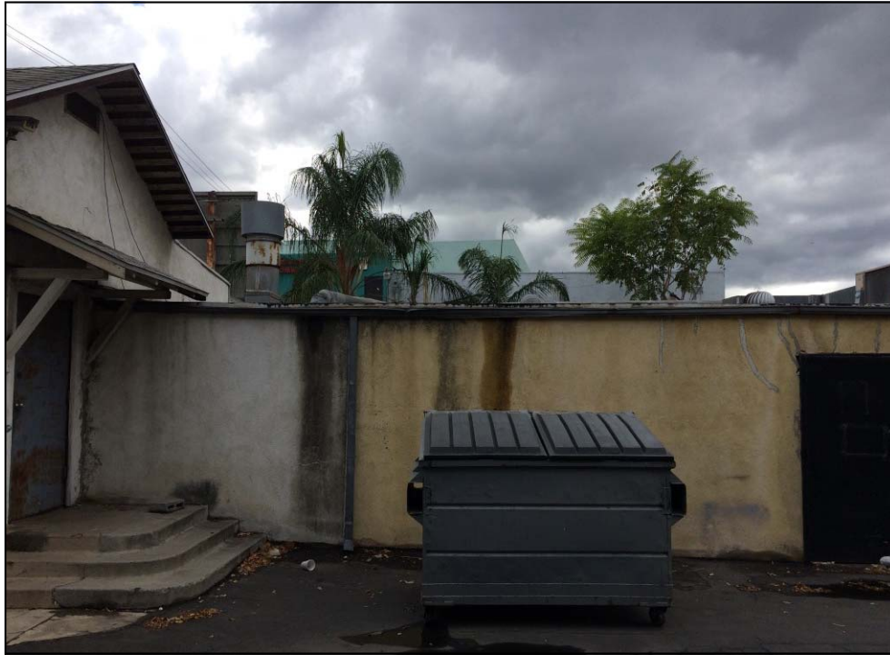
Photo 5: View of trash dumpster and water damage.
