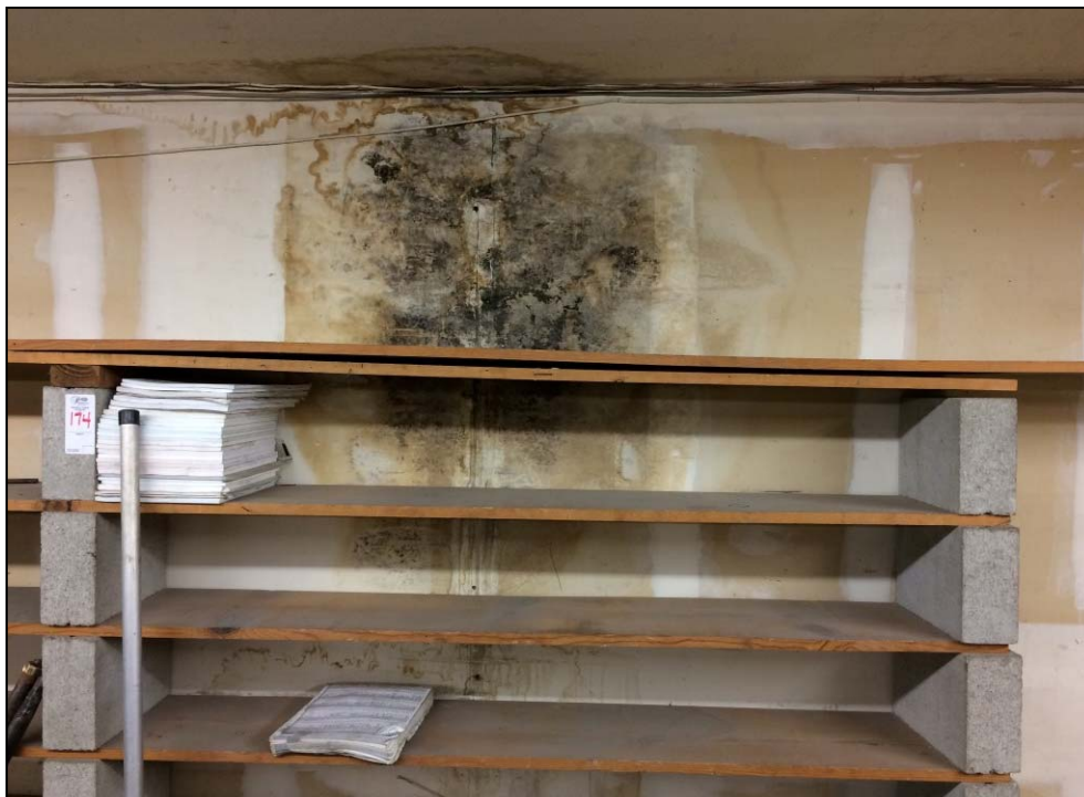
Photo 22: View of suspect mold growth within storage building.
