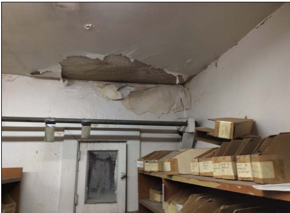
Photo 12: View of water damage within the interior portion of the two-story building.
