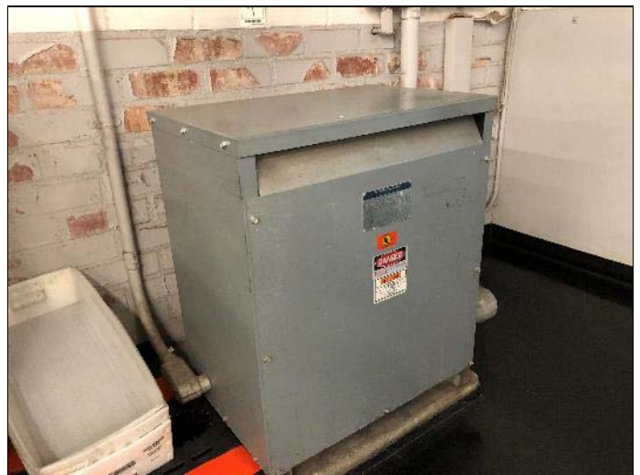
12. View of interior transformer.
