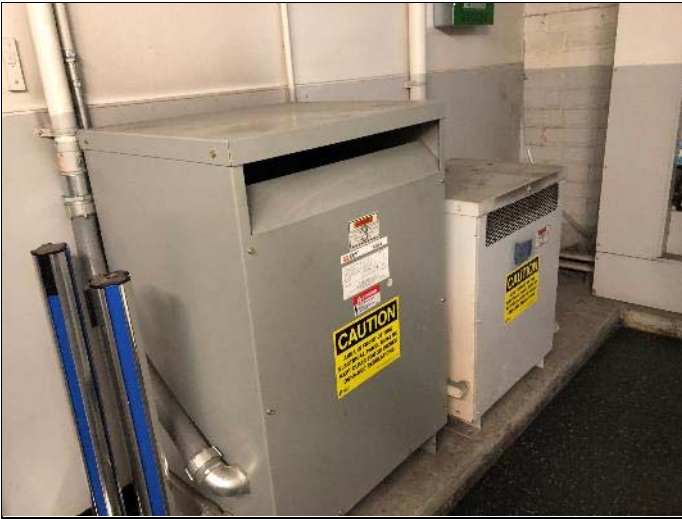
13. View of additional interior transformers.
