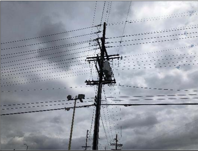
19. View of pole-mounted transformers.
