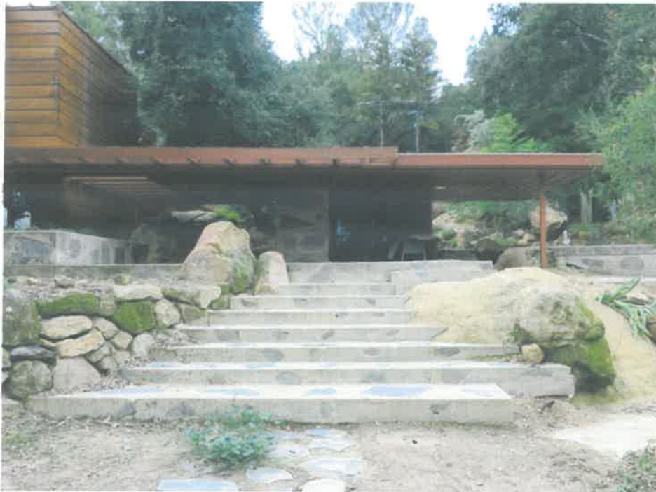
View west of the carport/entrance canopy and concrete steps with embedded stone (ARG, 2019).
