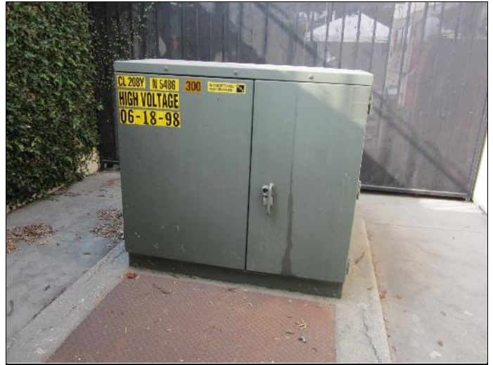
20. Pad-mounted electrical transformer on the subject property.
