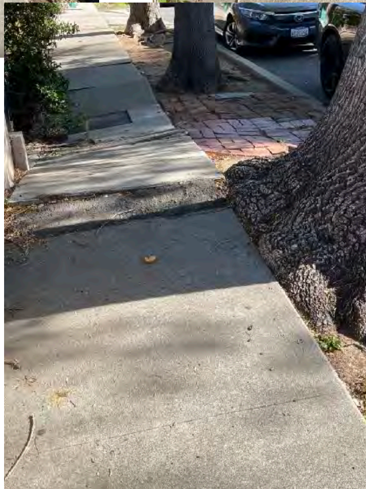
PHOTO 5 - TREE #2 - Raywood Ash ( Fraxinus angustifolia ) street tree #2 damage to sidewalk and curb. 1854-1860 Pandora Ave
