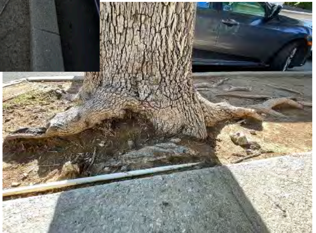
PHOTO 9 - Raywood Ash ( Fraxinus angustifolia ) street tree #4 damage to sidewalk and curb.
