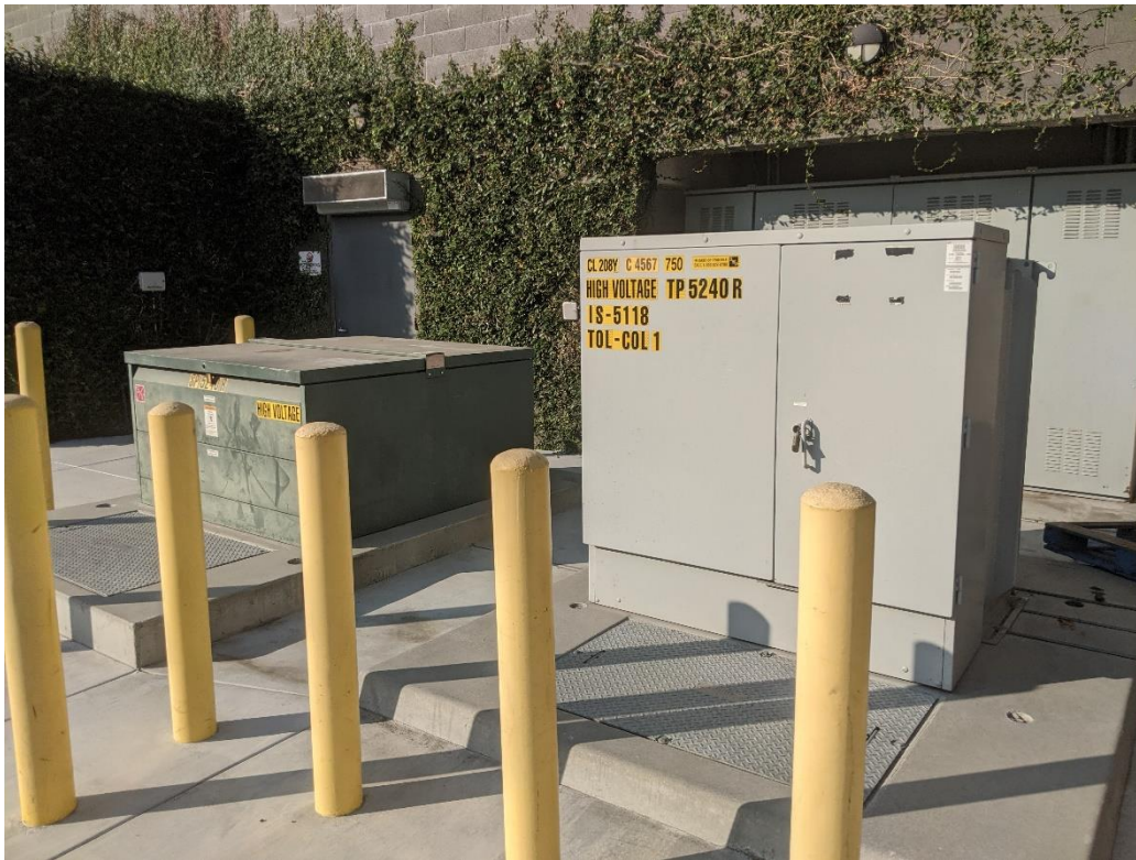
Two transformers maintained by the LA DWP on the east side of the subject property. 5240 Lankershim Boulevard, North Hollywood, California 91601
