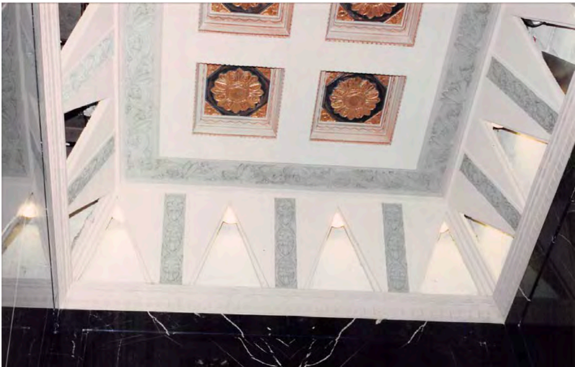
1990s: First-floor lobby grand entrance ceiling, uncovered during restoration (photo courtesy of the De Pietro Family)
