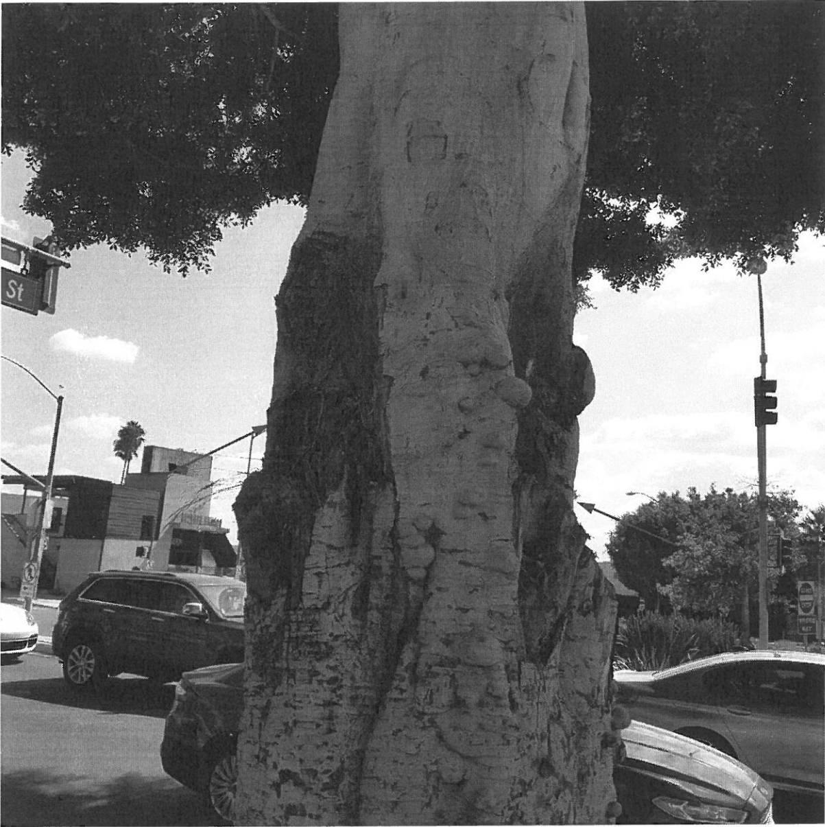
Looking southeast – red arrows at two old scaffold failures shown above
