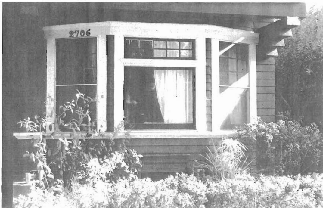
West façade detail: West slant bay paired nine-over one casement windows flank central fixed pane topped by ten light fixed transom, viewed to east.
