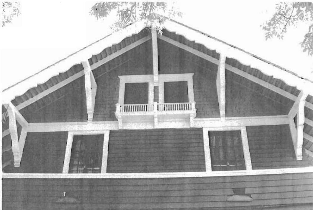
West façade detail: Corbel eave and bracket supports, shaped bargeboard, paired windows in gable end with bracket supported balcony with rail, full length overhanging balcony at second level with two pairs multi-paned French doors, viewed to east.
